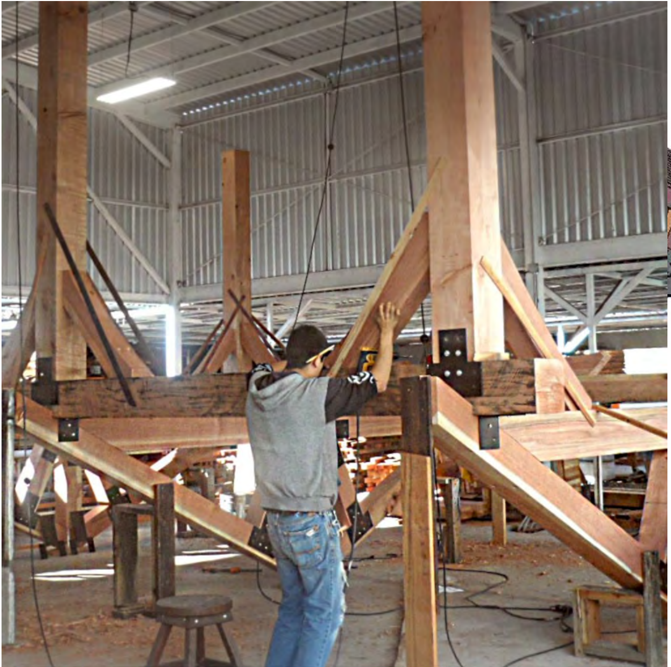
The Thick Timber Toledo Wood Pavilions. Construction image highlights massive timbers and steel plating used and shows Pavilion partially completed and prior to sanding or sealing. Yes, we build them upside down - much easier this way!
