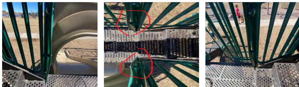
The playground seems to have shifted causing the supports to bend
